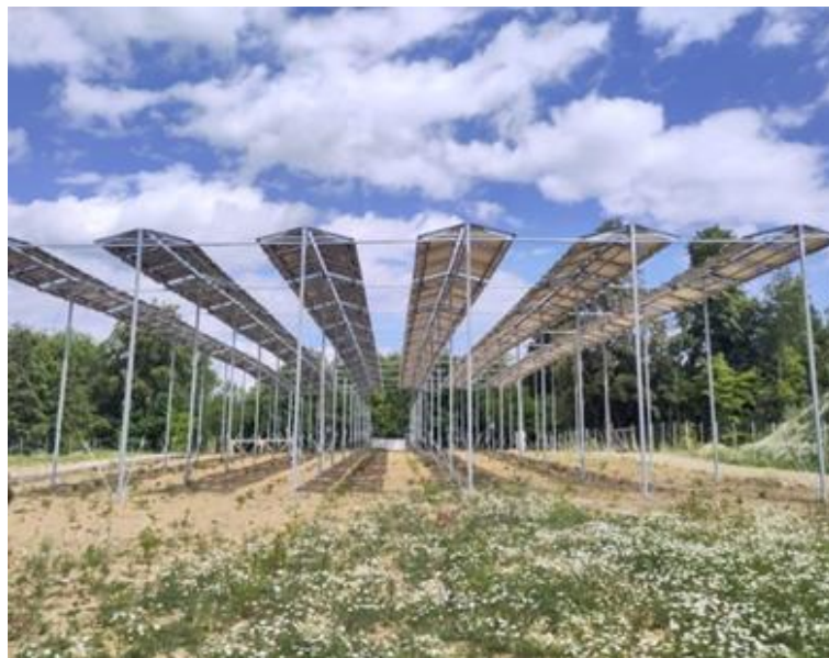
Picture: Photovoltaic system with an output of 135 kilowatts
